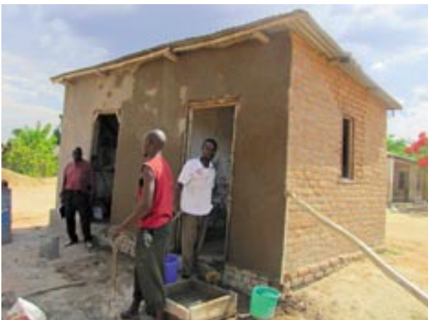
Office at Chitundu primary school being worked on as a result of an action point
